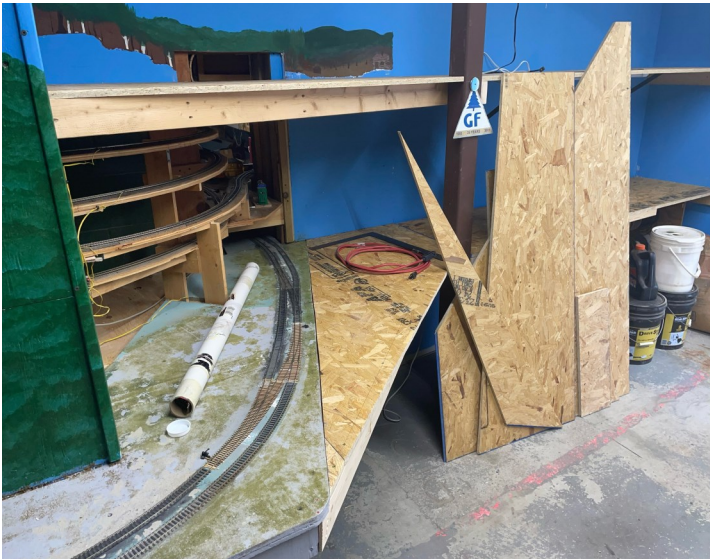
Reconfiguration of the staging yard entrance to accommodate the Seaport. The upper level will be the new SLR staging yard.
